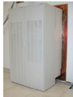
Figure 3. Filter Control Cabinet
