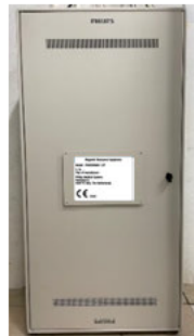
Figure 2. General Mains Distribution Unit
